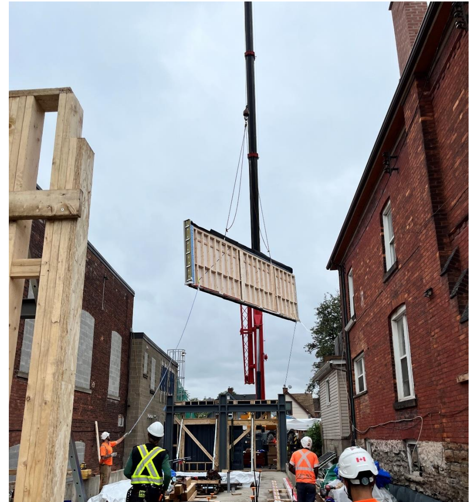
Photo courtesy of Assembly Corp
