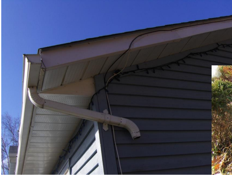
Downspout Missing or Damaged
