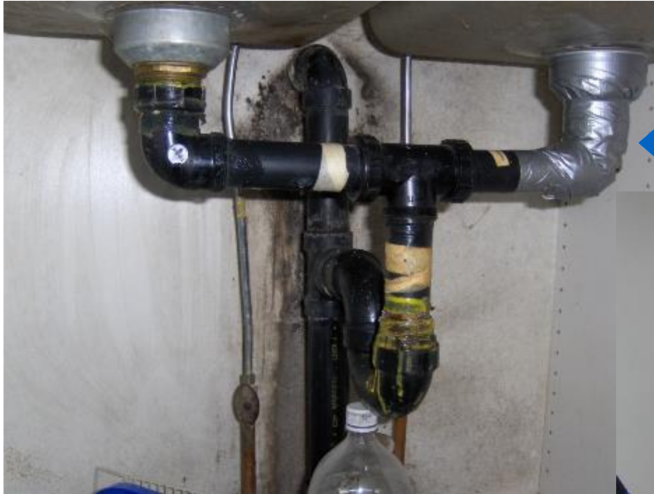
Under counter plumbing
