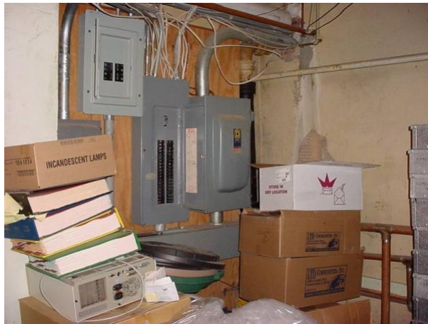
Electrical panel blocked by storage
