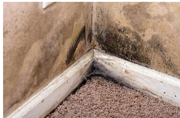
Interior mould caused by leaks
