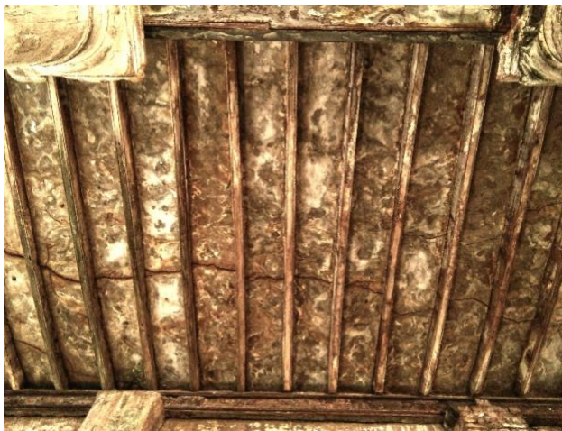
Dampness penetration leading to timber defects
