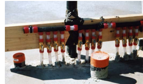
Slab hot water radiant heat distribution system
