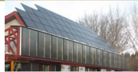
Solar hot water collectors
